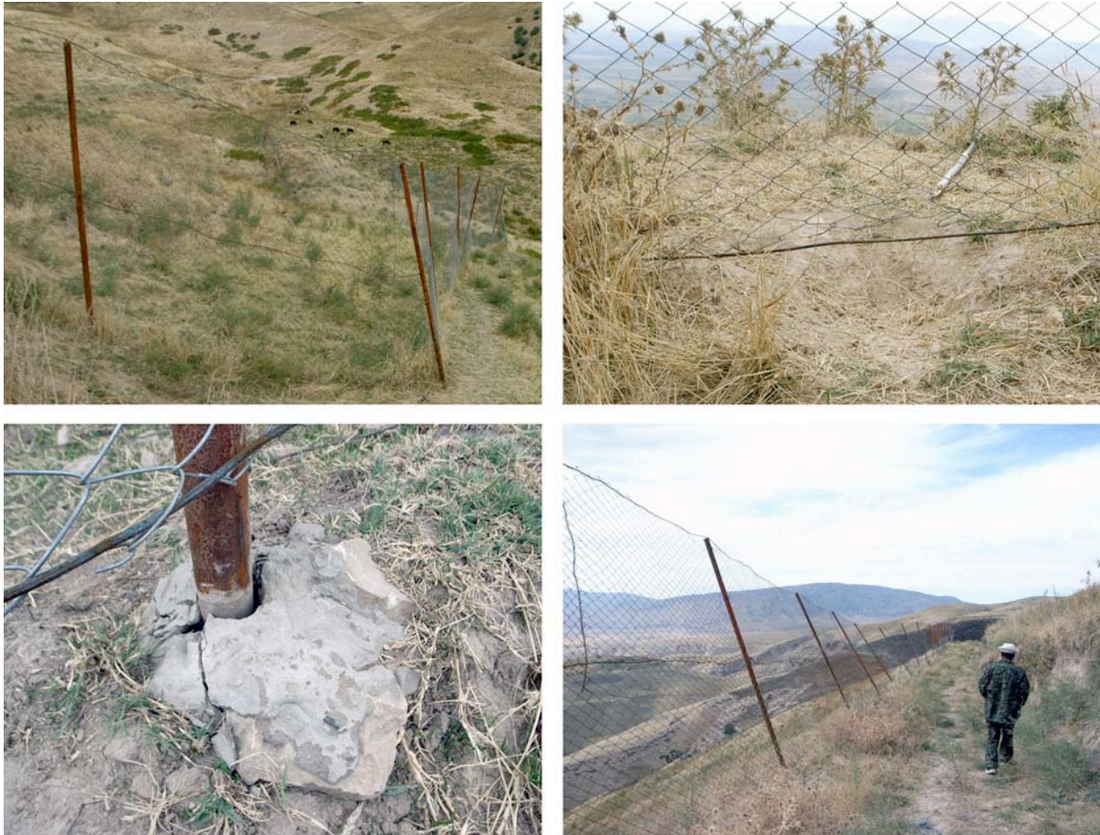
Plate 3. The unachieved perimeter fence of Nurek’s large enclosure presents serious structural flaws. Clockwise starting from upper left corner; a) Corner posts are not reinforced with power arms and stretchers; b) The fence is not buried in the ground allowing animals to easily dig their way through; c) The fence sinks at several locations and d) Concrete footing of posts is inadequate to uphold this 3-m high fence. Nurek’s large enclosure, Khatlon Province, Tajikistan, 30 September 2010. Photos ©Stéphane Ostrowski.
